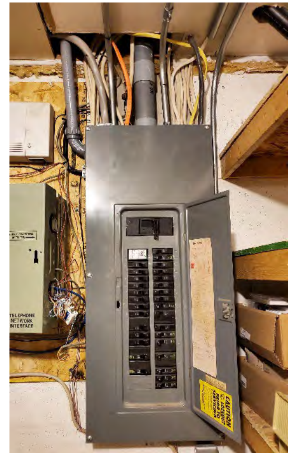
Figure 1: Existing Main Panelboard with Exposed Nonmetallic Cable
