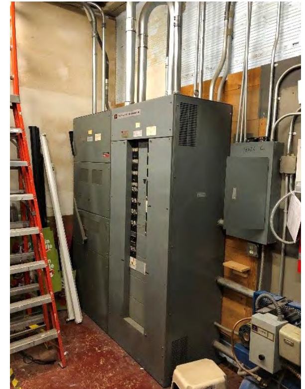
FIGURE 1: Main Electrical Service Equipment
