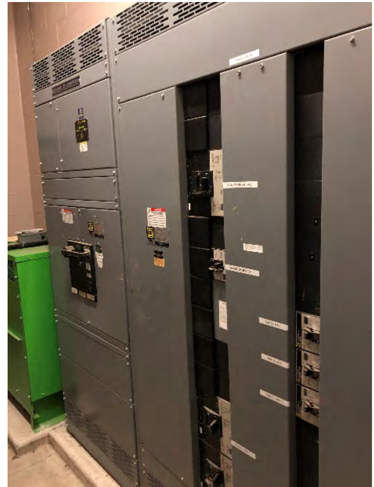
Figure 1: Existing Main Switchboard
