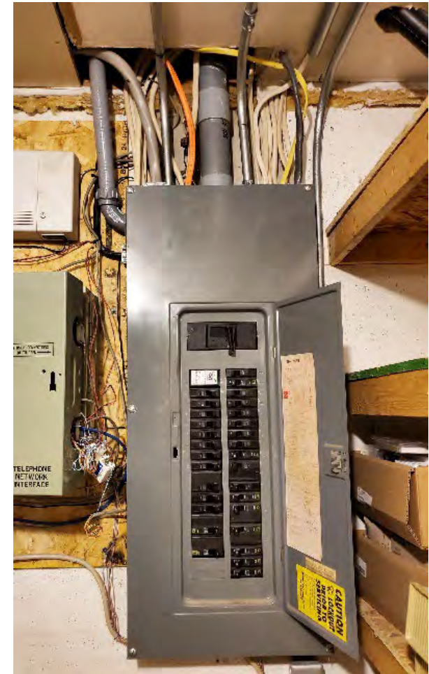
Figure 2: Existing Panelboard that May have Exceeded its BOMA Useful Life Expectancy
