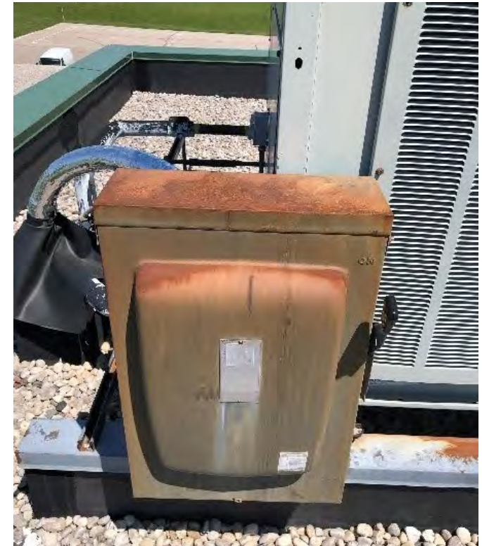
FIG 3: Disconnect switch on rooftop showing signs of major degradation
