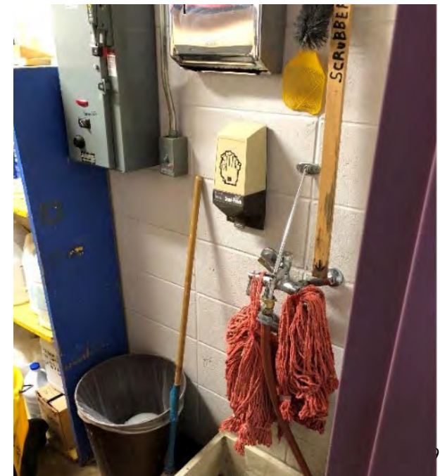
Figure 2: NEMA 1-Rated combination motor starter/disconnect switch adjacent to washdown/mop sink
