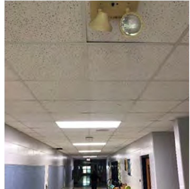
FIG 6: Typical hallway ceiling emergency light
